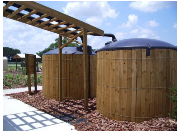
A rainwater harvesting cistern used for irrigation.
